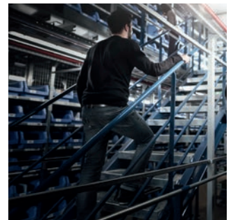
Railings and fall protection offer maximum safety for personnel and picked goods.
