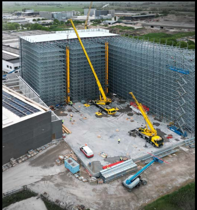
The new high-bay warehouse under construction: an area of 2,500 m 2 will soon provide space for 22,000 pallet locations.
