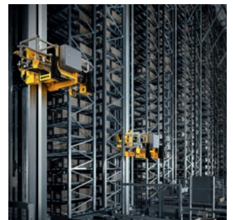
Automatic small parts warehouses are the first choice for high-performance environments such as spare parts stores and distribution centres.
